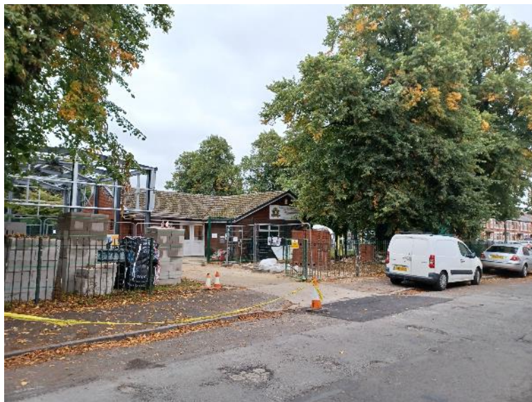
Existing centre with works taking place to the left to implement previous planning consent
